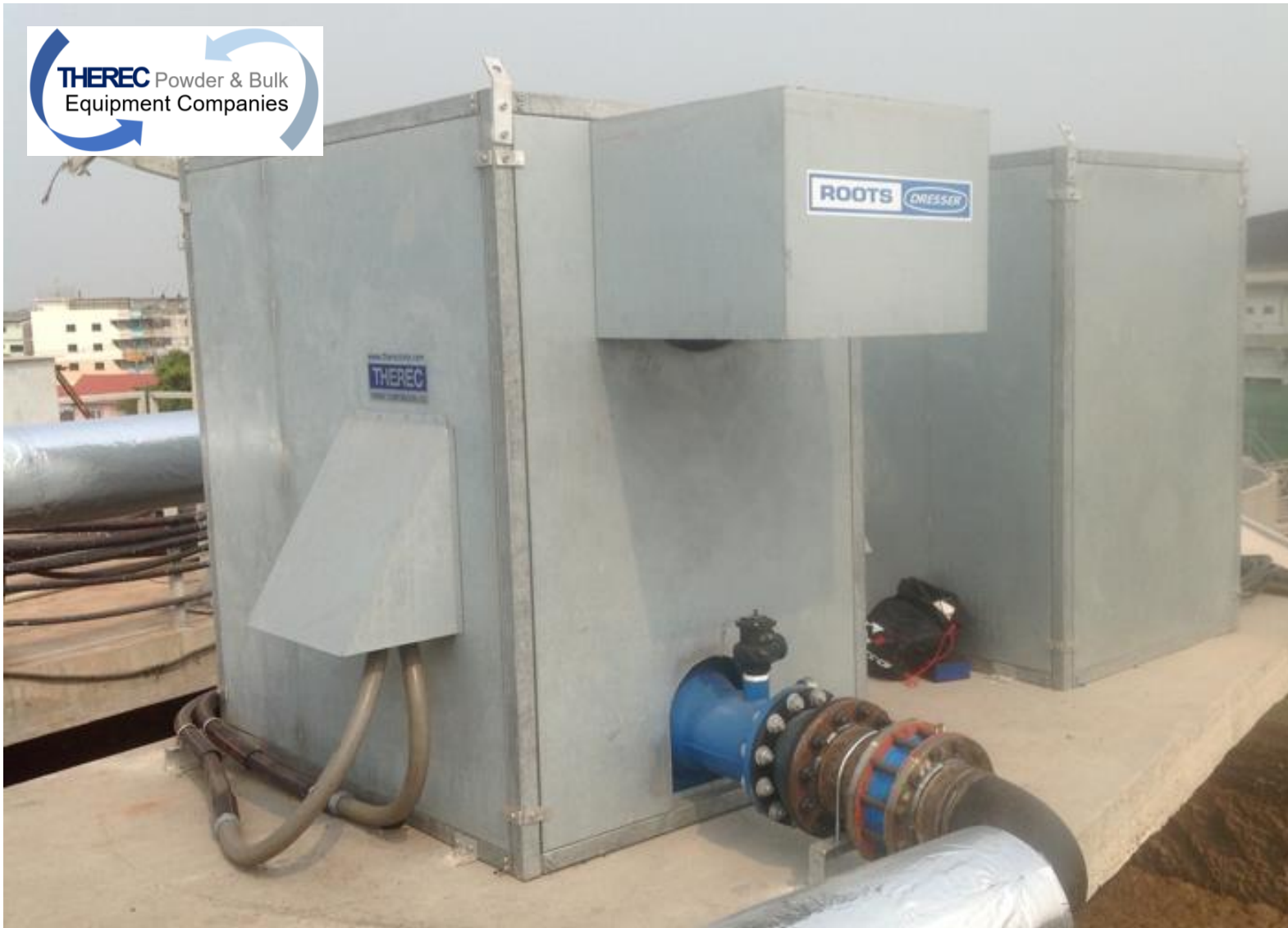
Union Frozen Product Co., Ltd., Samuthsakorn Plant 2014 / Dresser Roots Blower (Galvanized steel sheet + Hot dip galvanized frame)
